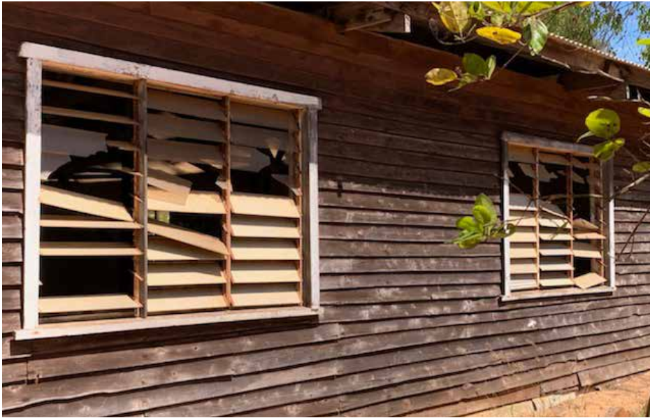
The windows of the church all need to be replaced.
